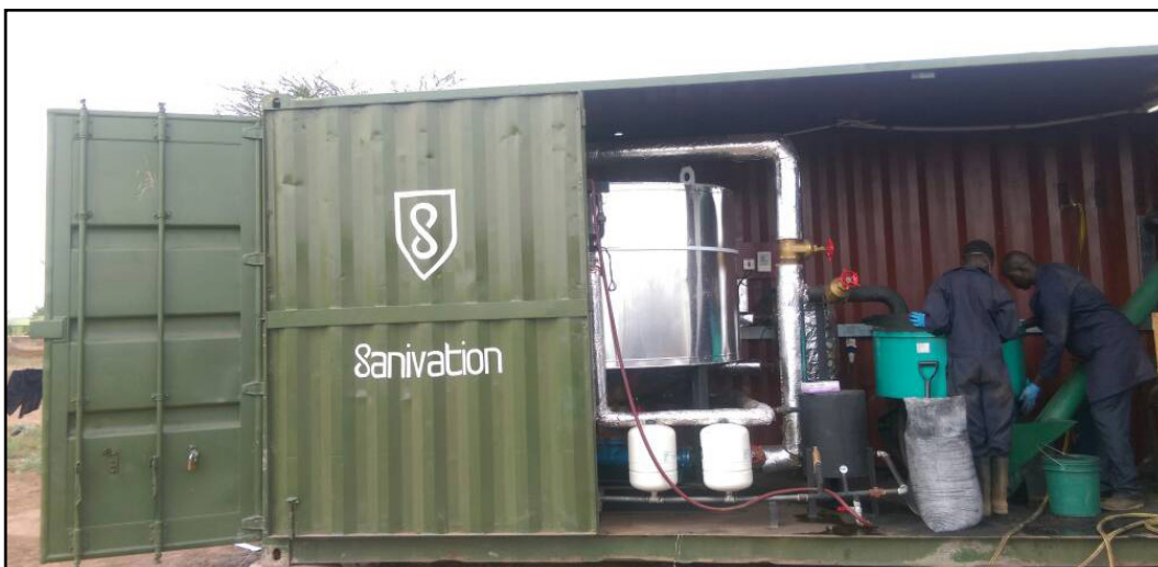
Sanivation's shipping container waste processing system used in Kakuma refugee
