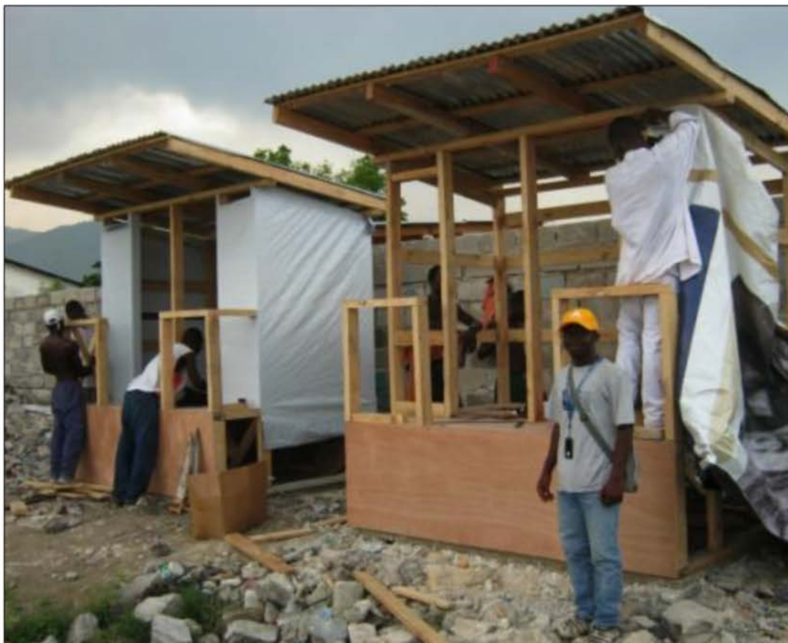
Wooden frame with plastic sheeting or rice bag walls – design for an IDP camp post disaster. Photo: SOIL
